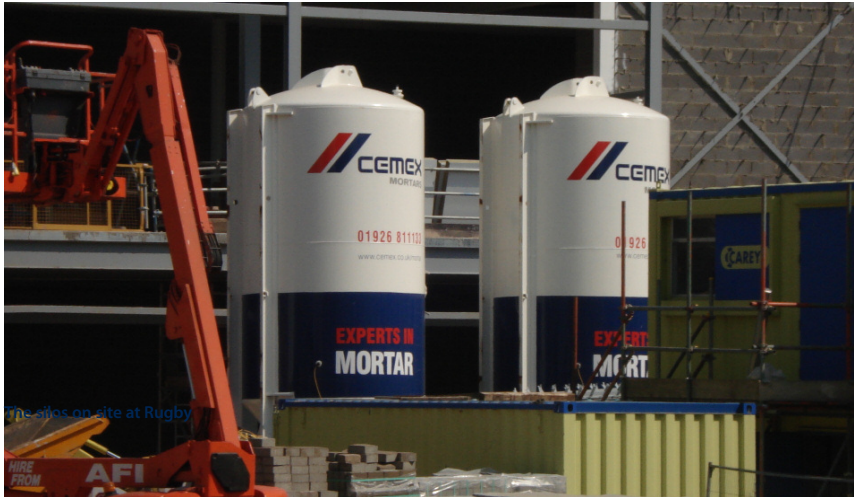
The dry mortar silos on site at Rugby
